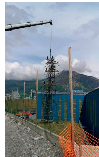
Removal of a pylon on the site in the aim of laying the electrical cables underground
